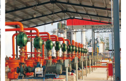
Oval gear flowmeter in petrochemical industry
