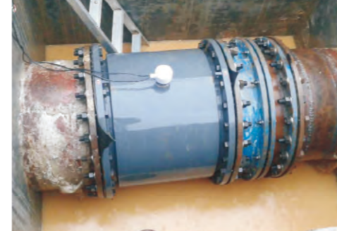
Magnetic flowmeter in under well field
