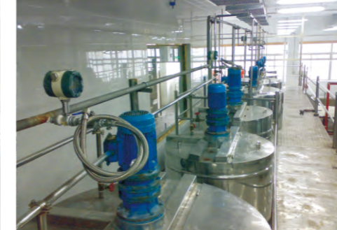
Liquid turbine flowmeter in food and beverage industry
