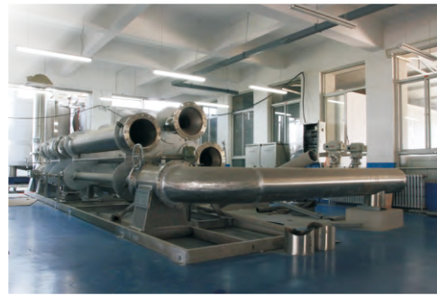
Liquid Calibration Facility
