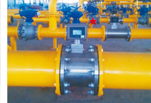
Gas turbine flow meter in nature gas filling field
