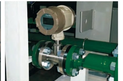
Liquid turbine flowmeter in water supply plant
