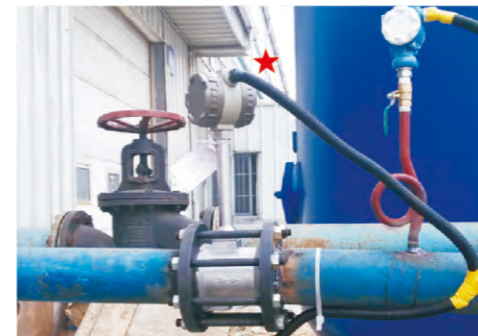
Vortex flowmeter in oxygen measurement
