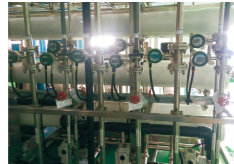
Turbine flowmeter in water supply field
